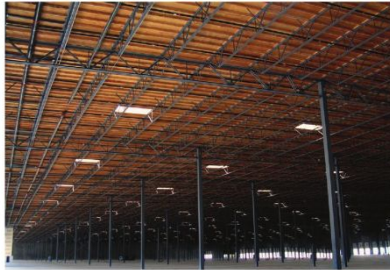
Type I: 111,484-m 2 (1.2 million-sf) panelized roof system using interior FRT lumber and plywood in Phoenix, Arizona.
