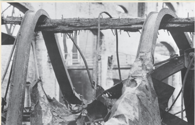
In 1953, a fire in a casein glue factory demonstrated the superior fire-endurance of untreated wood over steel.
